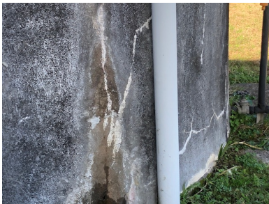
Cracked water tank that no longer holds water, on Italia Road, Balickera
